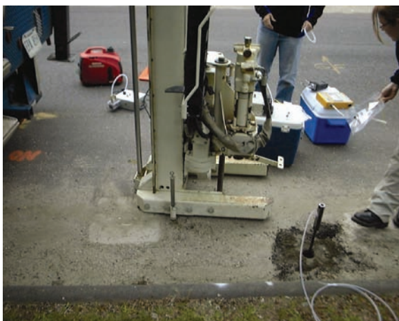
Figure 22. Proximity of dedicated vapor probe (metal cover surrounded by white concrete at base of Geoprobe unit), PRT, and GVP sampling systems.
